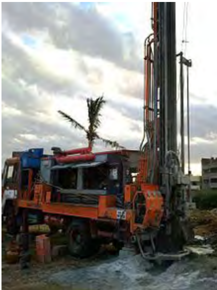
Rig drilling popularly known as 'PD series' in operation for Water well drilling, in India.
