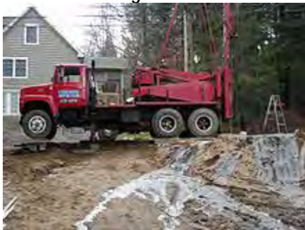
SpeedStar cable tool drilling rig, Ballston Spa, New York (Truck mounted Drill)
