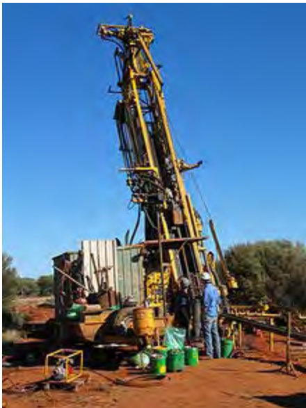
Multi-combination drilling rig (capable of both diamond and reverse circulation drilling). Rig is currently set up for diamond drilling.
